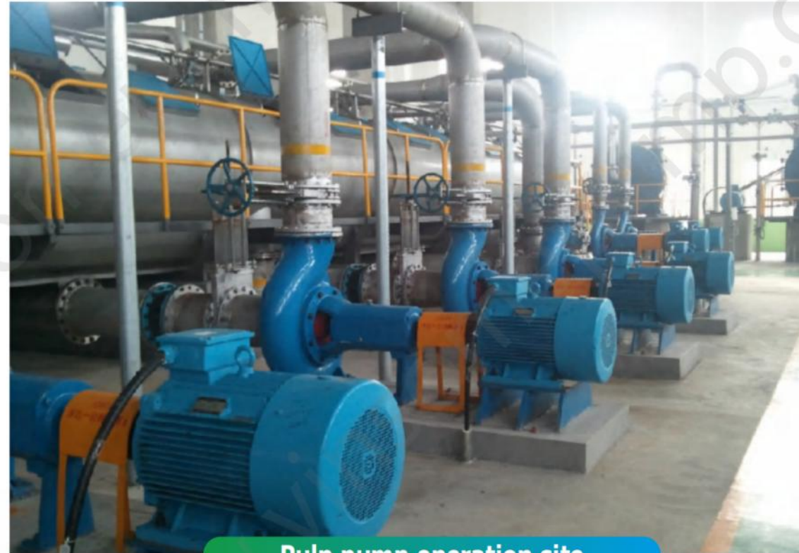
Pulp pump operation site
